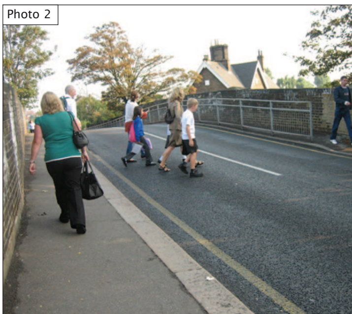
Far Left: Substandard pavement width with damaged guard rail.
